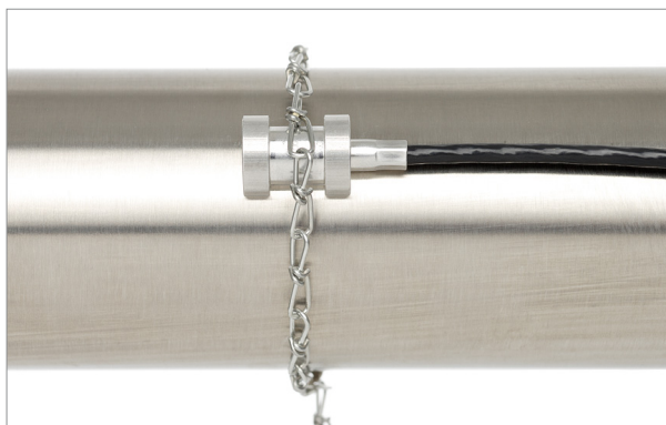
PT100 transducer fixed to pipe
