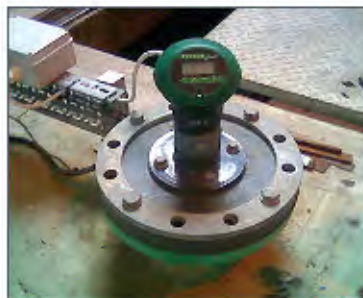
IMP ON A LIQUID LIME TANK
