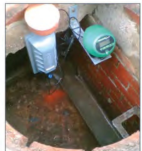
IMP MONITORING IN A CSO CHAMBER
